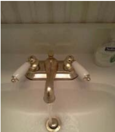
MB- drain plug does not operate
