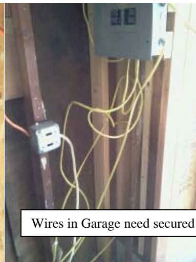
Splice in Garage Needs Junction Box
