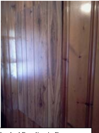
Patched Paneling in Den area
